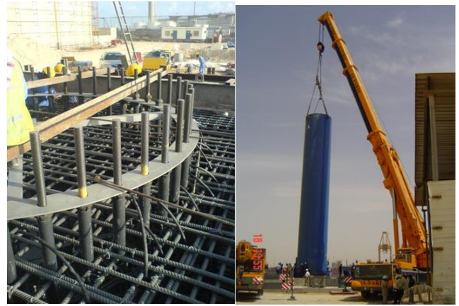
Tie Down Bolts - Jebel Ali Crane Base, Dubai
